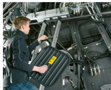
Many attachment points for the mobile ladder.
